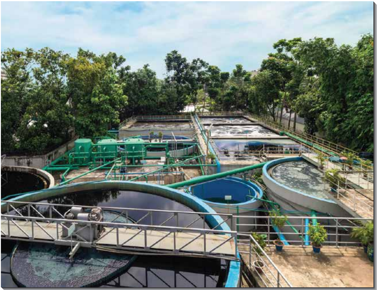
ETP Plant for Safe Environment
